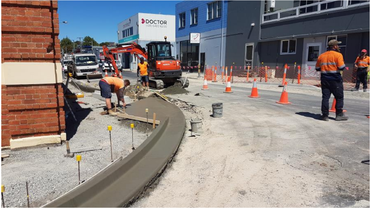
1.10 Renewal of the section of Clayton Drive, east of Hillwood Rise is complete.
