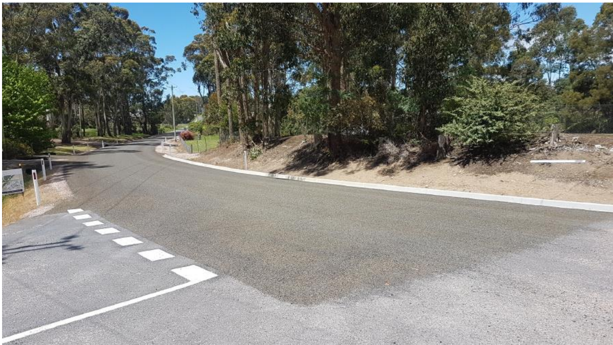
1.11 The upgrade of the Cenotaph Car Park was completed in advance of Remembrance Day activities. This project was able to double the capacity of the car park but only increased the footprint by around 10%. The new layout provides better links to the Cenotaph and with the Coastal Pathway.
